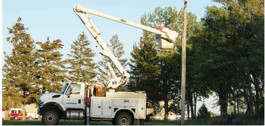
DEC Line workers disconnect the power making the accident scene safe to work.
